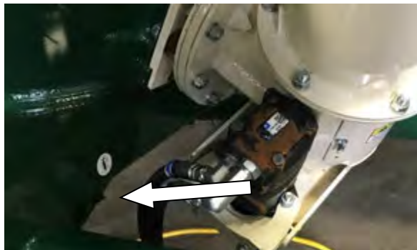
Figure 57 - Gearbox Lubrication Upper Bearing Remote Location.
