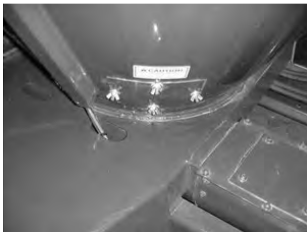
Figure 21 - Tank Cone Clean-Out Door On Right-Hand Side.
