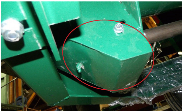
Figure 84 - Vertical Auger Bevel Gears Shield.
