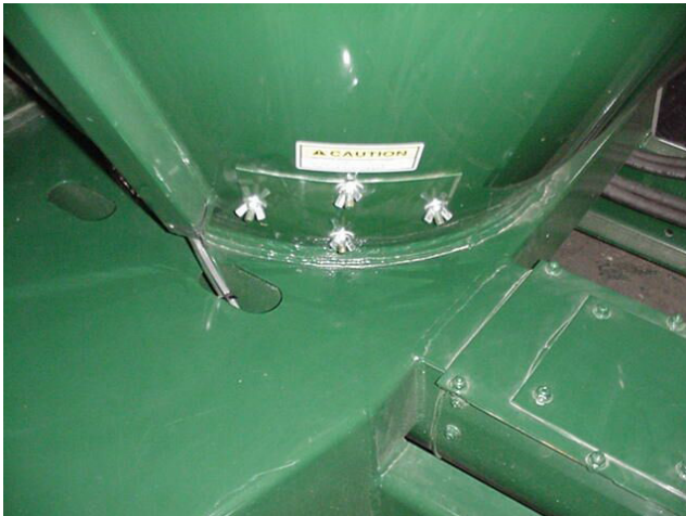
Figure 123 - Tank Cone Clean-Out Door On Right-Hand Side.
