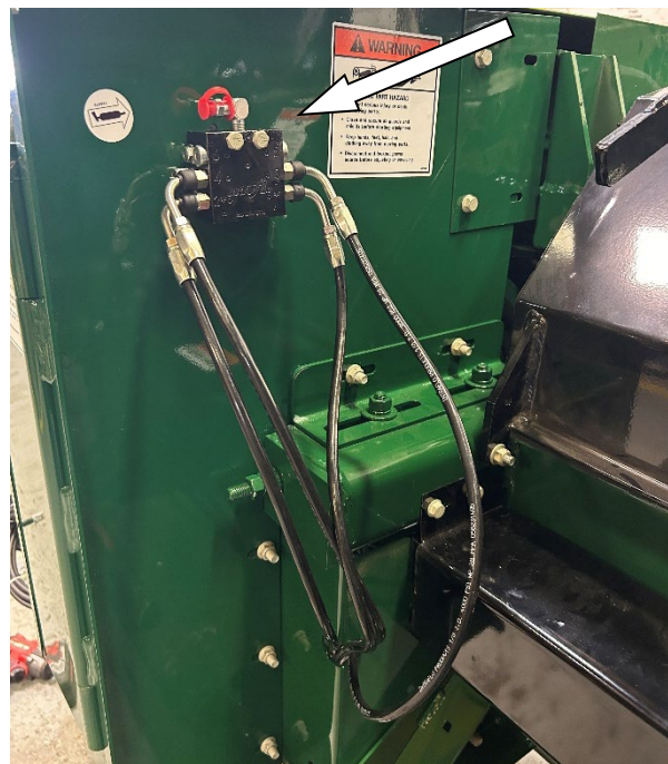
Figure 69 – Remote Greasing block.
