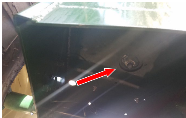
Figure 112 –Drain Underneath Reservoir Tank Base (Red Arrow).
