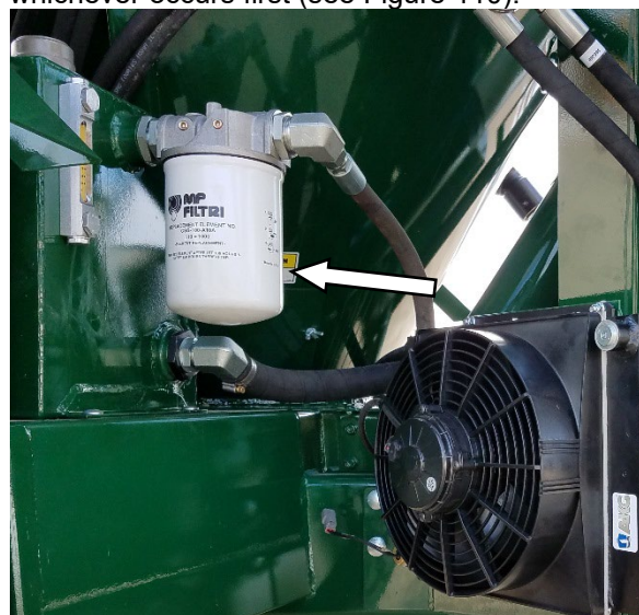
Figure 110 – Reservoir Filter (see Arrow)
