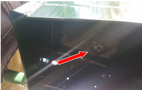
Figure 112 – Drain Underneath Reservoir Tank Base (Red Arrow).
