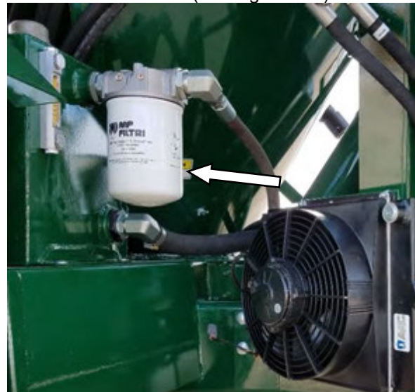
Figure 110 – Reservoir Filter (see Arrow)
