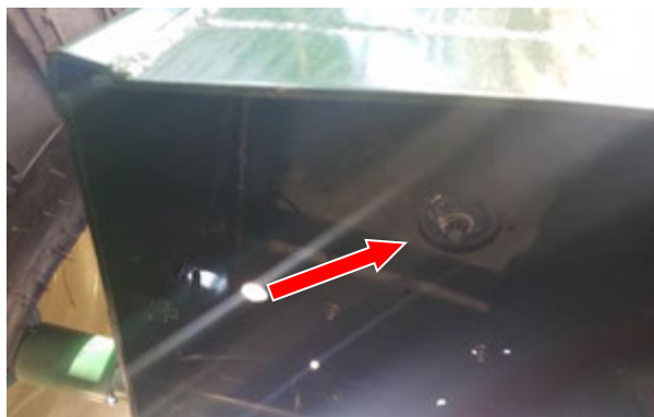
Figure 112 –Drain Underneath Reservoir Tank Base (Red Arrow).
