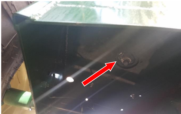
Figure 98 – Drain Underneath Reservoir Tank Base (Red Arrow).
