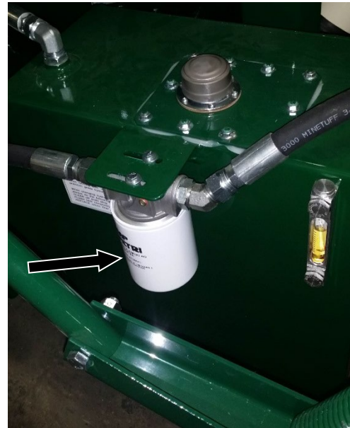
Figure 75 – Reservoir Filter (See Arrow).
